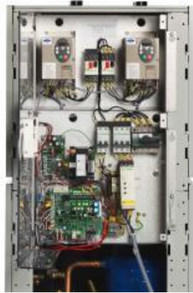
Electrical cabinet open
